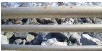
Photo: Maintenance Cleaning of tea-staining of hand railings on the sea side
